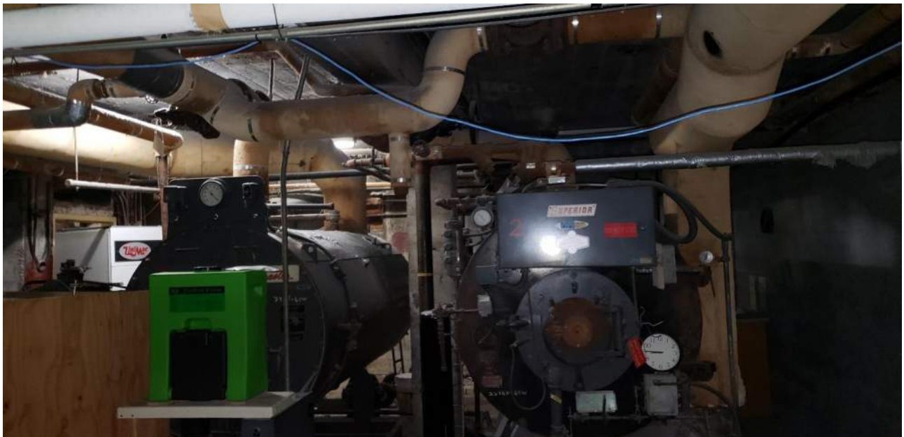
1920's Boiler Room
